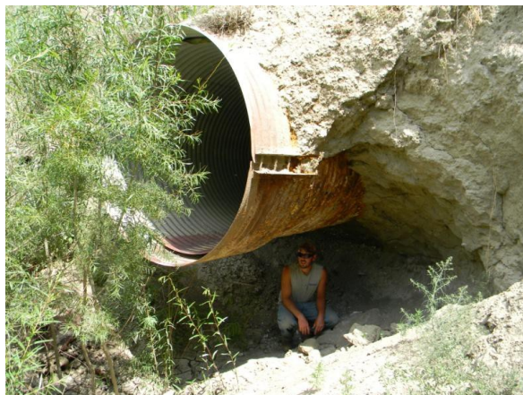
A culvert contributing to erosion in William Coulee, tributary to the Musselshell near Fort Peck Reservoir identified during BLM habitat inventory. Photo supplied by Jake Chaffin, BLM
