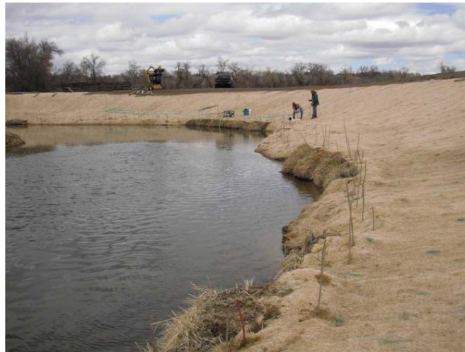
Cuttings and operation on Big Goose Creek (Project 4) Photo supplied by Carrie Rogaczewski, SCCD
